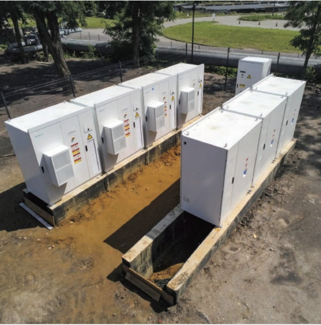
Bytom, Poland Battery capacity: 1505 kWh
