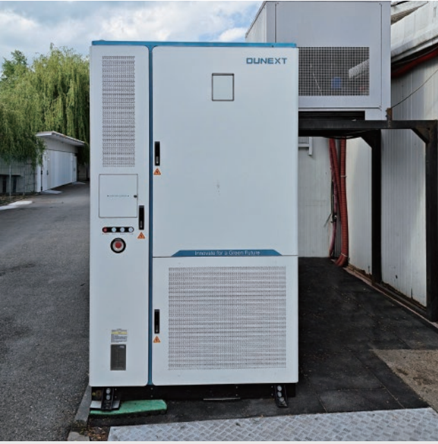
Targu Jiu, Romania Battery capacity: 233 kWh
