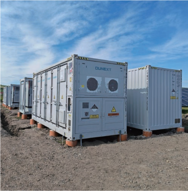
Cluj, Romania Battery capacity: 20 MWh
