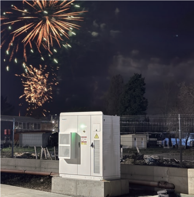
Pomorie, Bulgaria Battery capacity: 215 kWh
