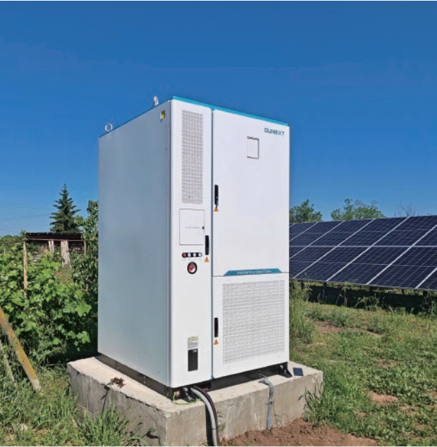
Village Borets , Bulgaria Battery capacity: 233 kWh
