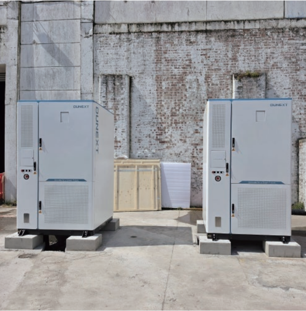
Wales, UK Battery capacity: 466 kWh
