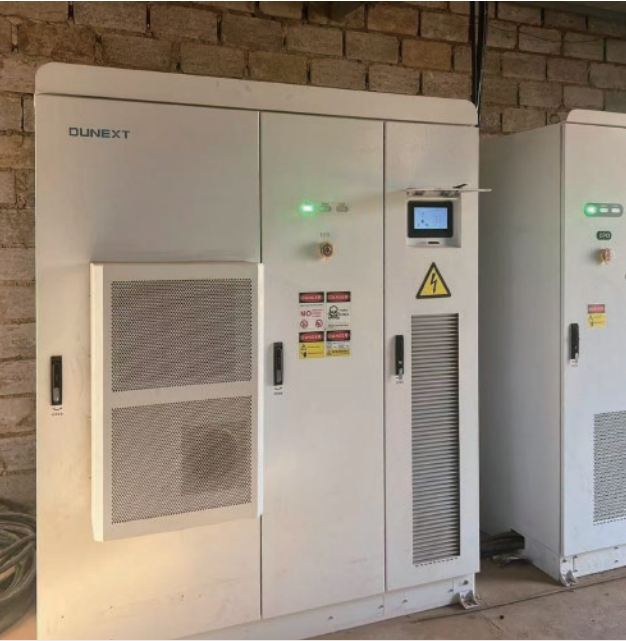
Kolwezi, DR Congo Battery capacity: 215 kWh
