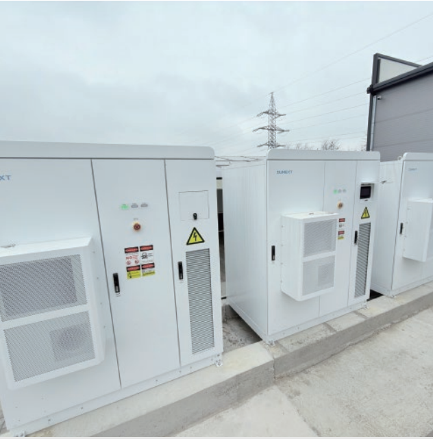
Suceava, Romania Battery capacity: 645 kWh
