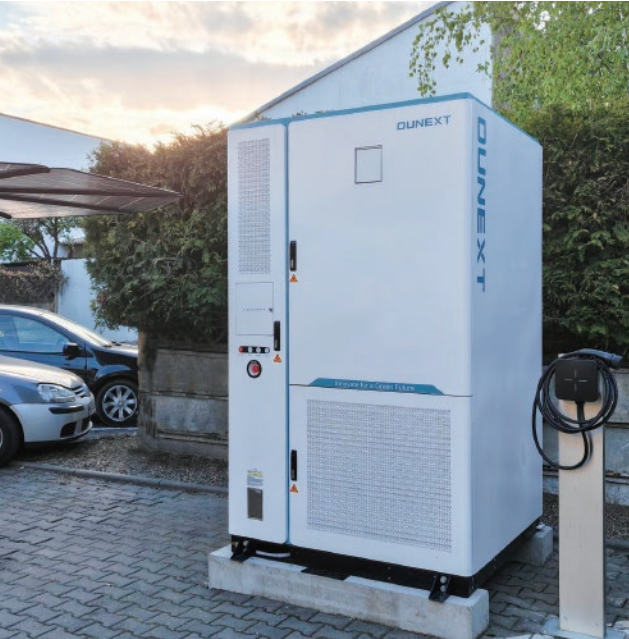
Targu Mures, Romania Battery capacity: 233 kWh
