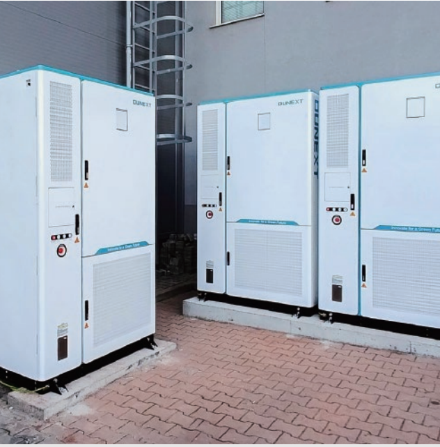
Sofia, Bulgaria Battery capacity: 699 kWh
