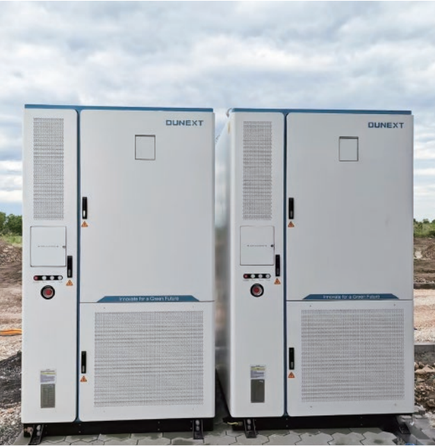
Targu Mures, Romania Battery capacity: 466 kWh
