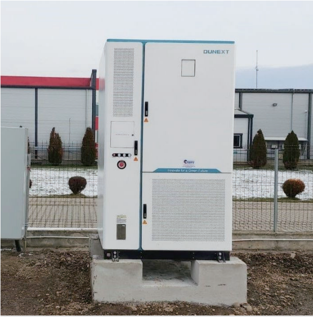
Sofia, Bulgaria Battery capacity: 233 kWh
