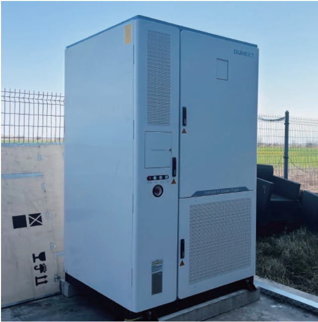
Plovdiv, Bulgaria Battery capacity: 233 kWh
