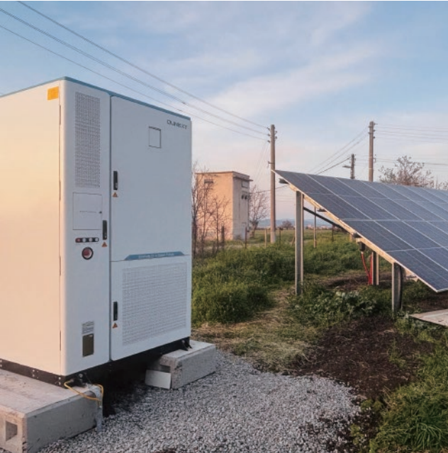
Voivoda, Bulgaria Battery capacity: 233 kWh
