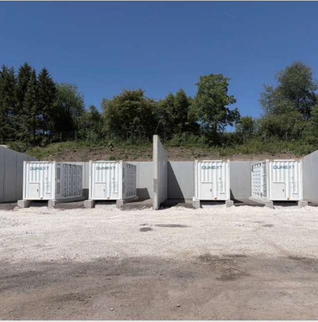
Schörfling am Attersee, Austria Battery capacity: 6 MWh
