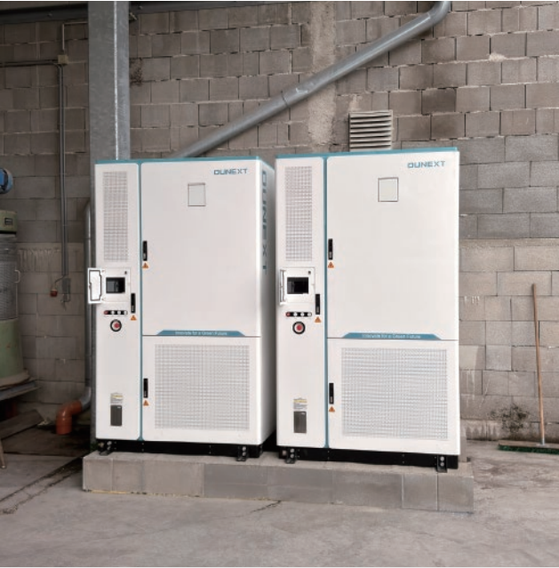
Groß-Schweinbarth, Austria Battery capacity: 466 kWh
