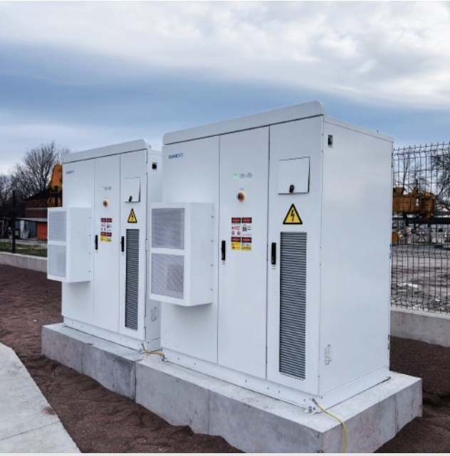
Pomorie, Bulgaria Battery capacity: 430 kWh
