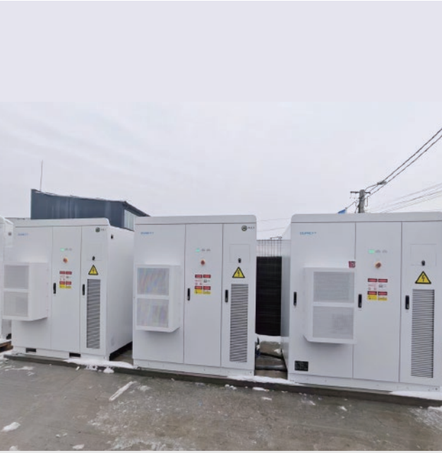
Targu Jiu, Romania Battery capacity: 645 kWh
