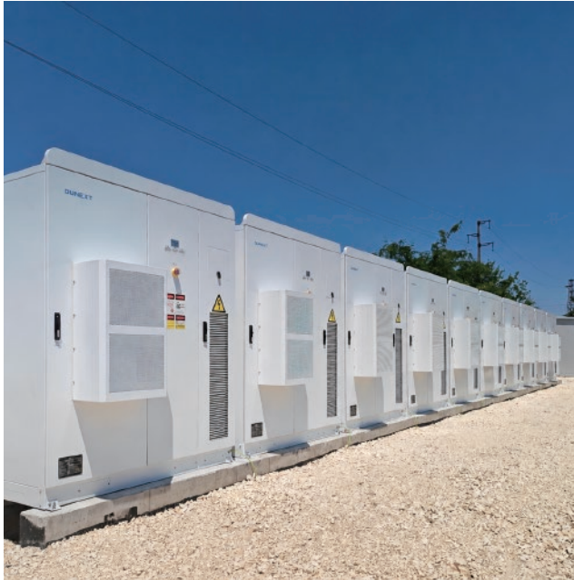
Tutrakan, Bulgaria Battery capacity: 2150 kWh
