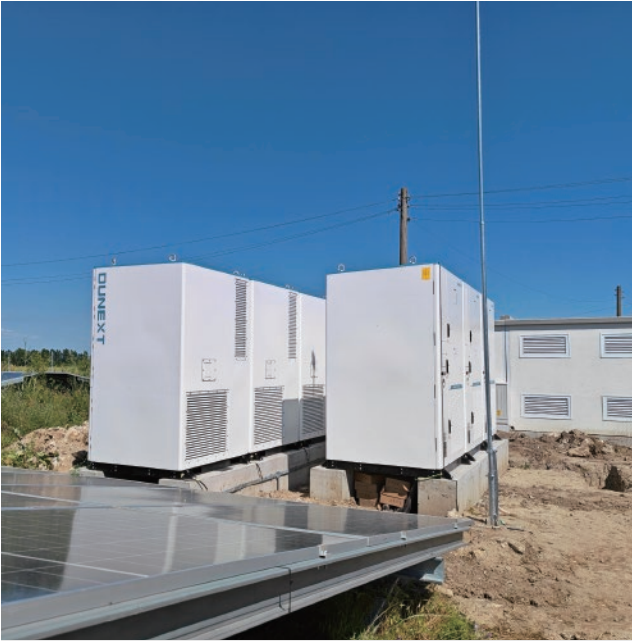
Plovdiv, Bulgaria Battery capacity: 1864 kWh
