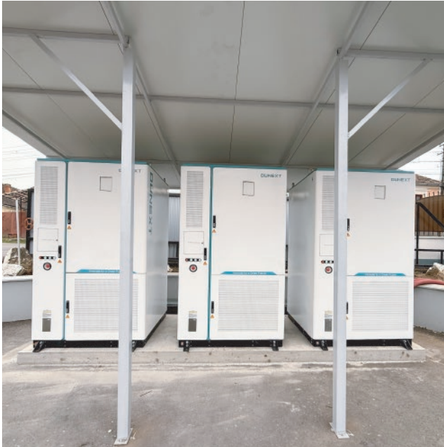
📍 Targu Mures, Romania 🔋 Battery capacity: 699 kWh
